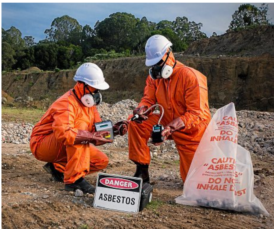
MINIMISING HARM: Ecoteam workers take a safety-first approach in high-risk work environments. PHOTO: CONTRIBUTED
